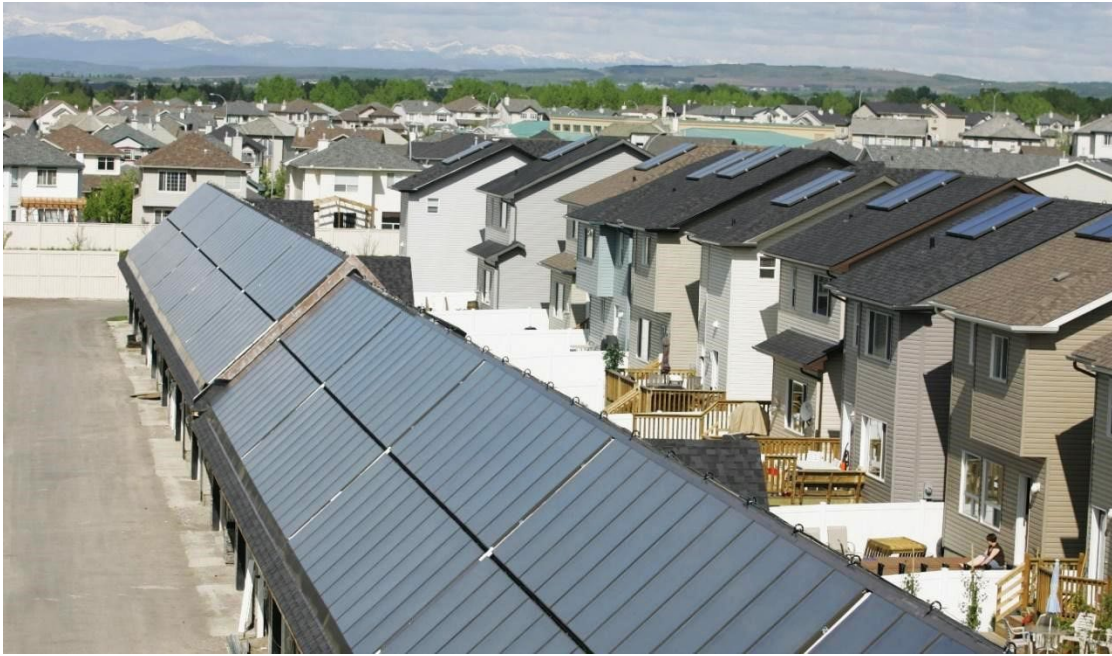
Figure 8: Houses and adjoining garages equipped with rooftop solar thermal collectors for hot water and space heating, respectively.
